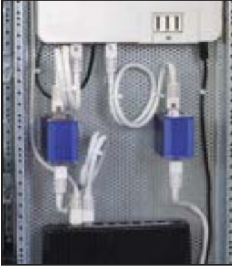
The protection of your equipment ethernet
